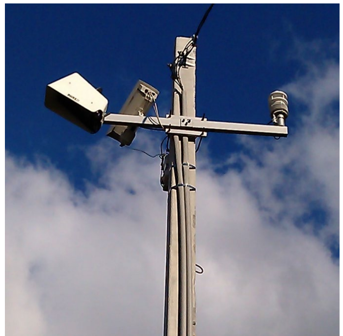
Slim yet powerful RWIS setup with a NIRS31 road sensor, a WS600 weather station, and a camera. Credit: OTT HydroMet
